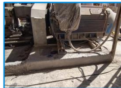
Acid Circulation Pump Chemicals
