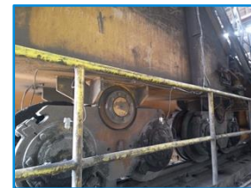
Casting Crane Steel Melt Shop
